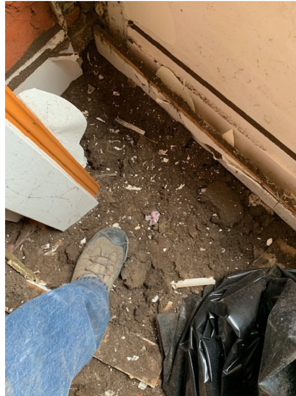
Waste on Floor Having Fallen from Ceiling
