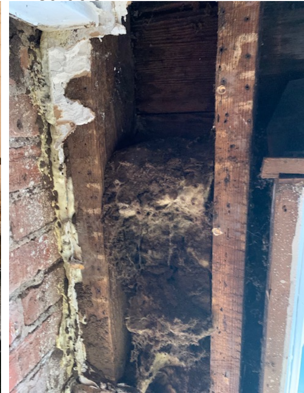
Waste compacted into the Wall Originally Behind Insulation
