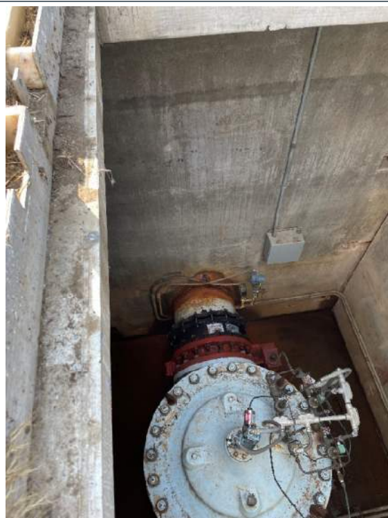
Photo 4-4-25 A&M - Albany Metering Vault – Rusty Piping
