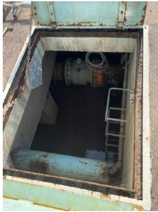
Photo 4-2-2 34 th St - Flow Meter Vault – Standing Water
