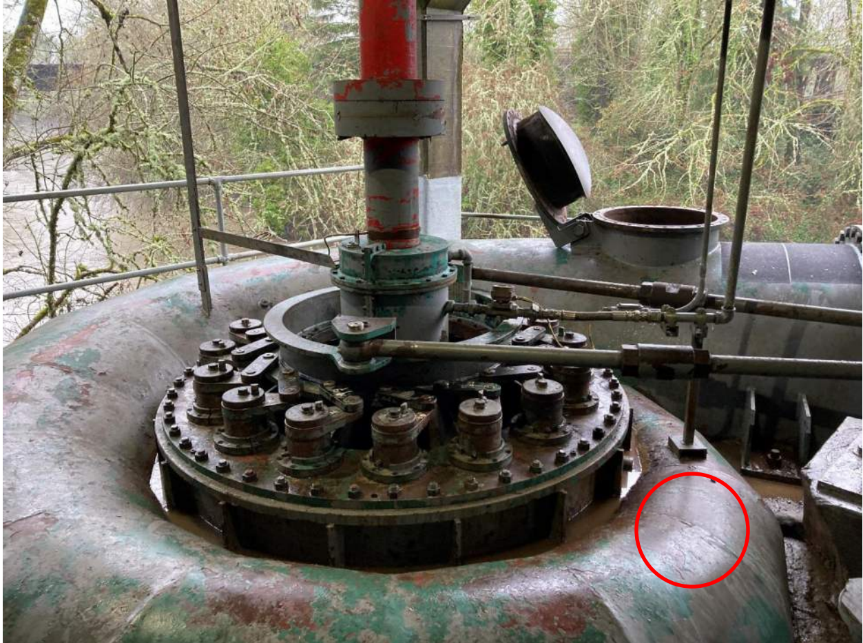
Figure 4. Approximate Location of the Recommended Cleanout Flange Location on the Spiral Case
