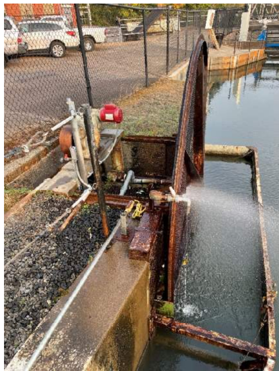
Photo 4-4-21 Vine St – RW Screen – Rust
