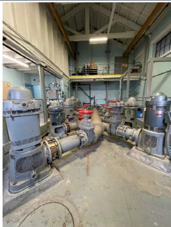
Photo 4-4-13 Vine St – RW Pump Station – Pipe Coating Aged
