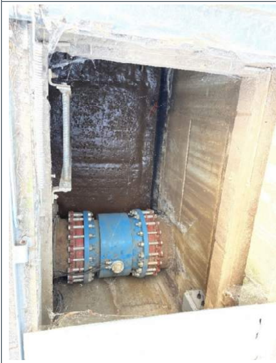
Photo 4-2-7 North Albany - Flow Meter Vault – Mud on Floor
