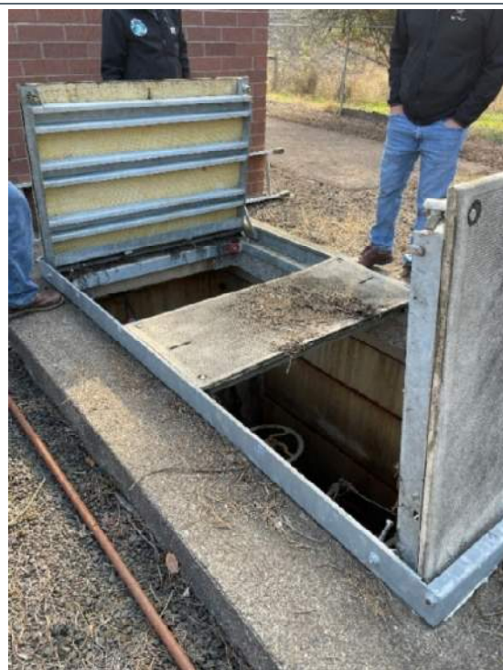
Photo 4-2-6 North Albany – Valve Vault – FRP Hatch
