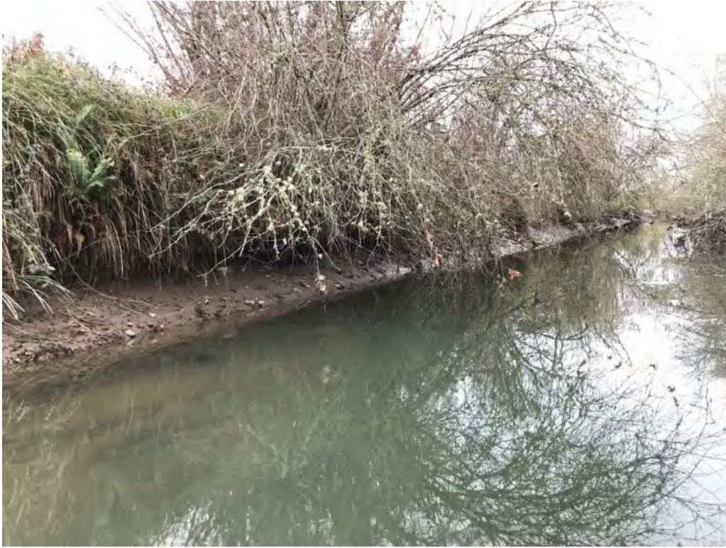
Photo 11. Erosion at the toe of the berm facing northwest.
