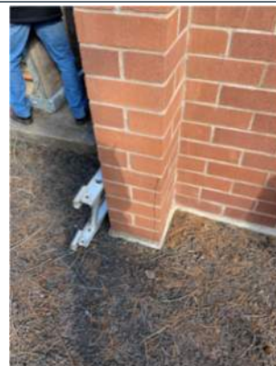
Photo 4-3-30 North Albany Pump Station
