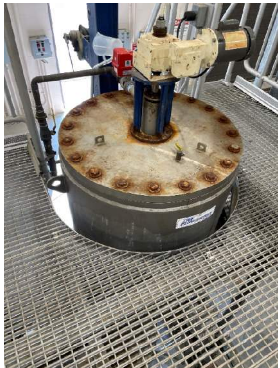
Photo 4-4-27 A&M WTP – Strainers – Rusty Disimilar Metals
