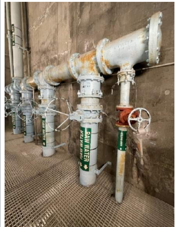
Photo 4-4-26 A&M Intake Structure – Piping Discoloration
