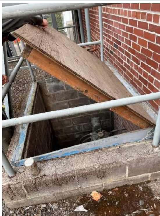
Photo 4-2-8 Vine St - RWPS Valve Vault – Wood Lid
