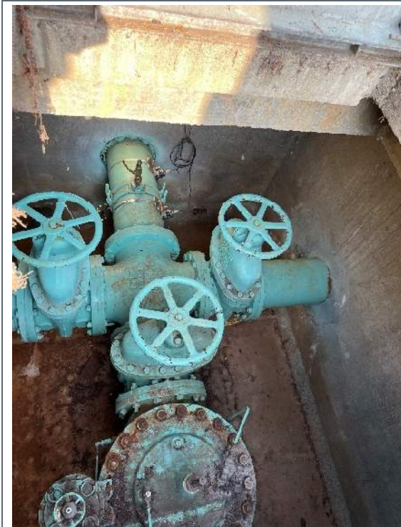
Photo 4-6-1 Wildwood – Ultrasonic Flow Meter
