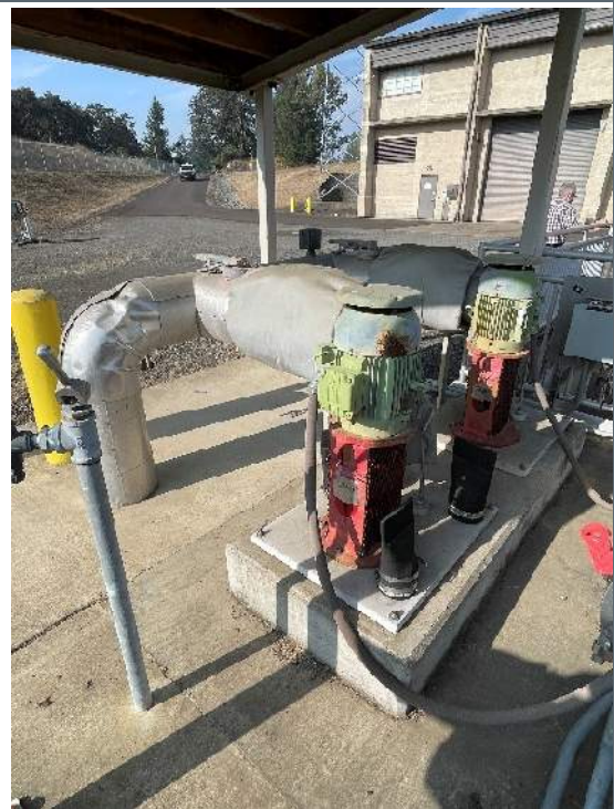
Photo 4-6-4 A&M WTP - Neutralization Basin – Outdoor Pumps
