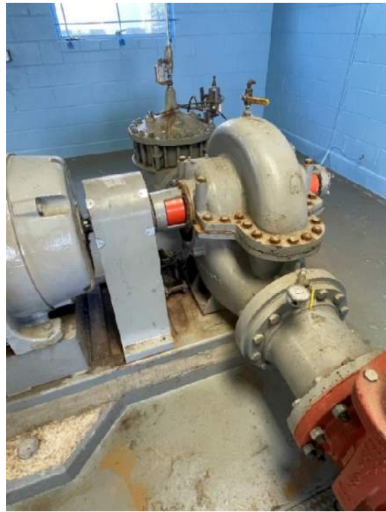
Photo 4-4-5 Maple PS – Pipe - Coating Damage
