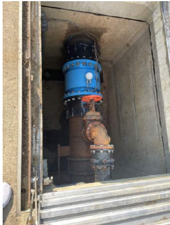
Photo 4-4-7 Maple – Valve Vault – Rusty Piping
