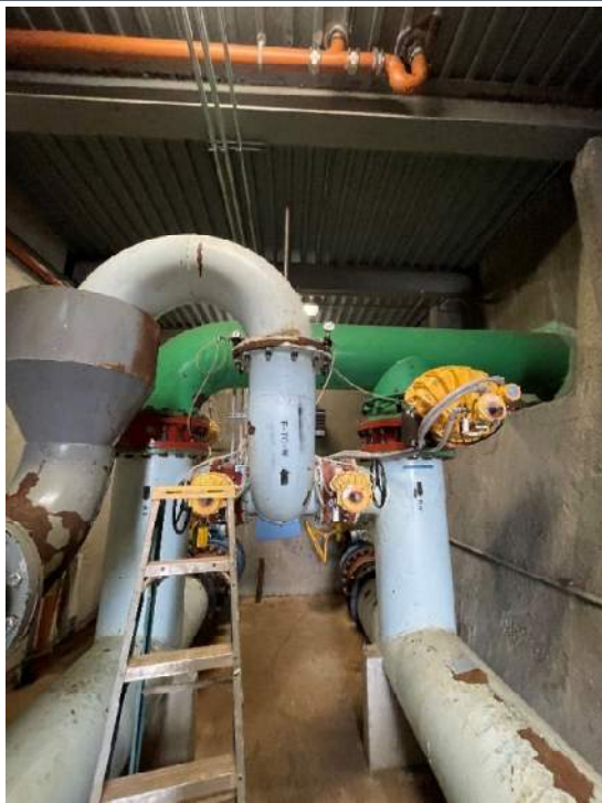
Photo 4-4-18 Vine St – Pipe Gallery – Corrosion & Rust
