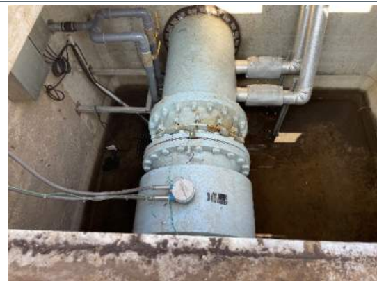
Photo 4-2-13 A&M WTP – ACH & Metering Vault – Standing Water
