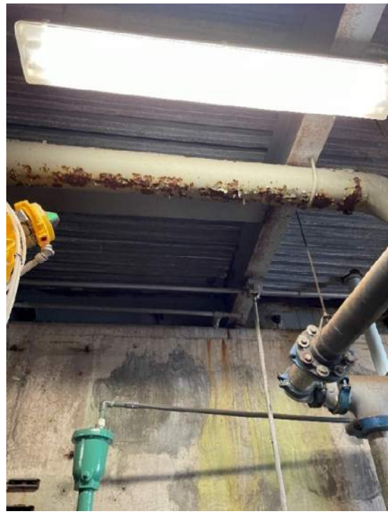
Photo 4-4-17 Vine St – Pipe Gallery – Corrosion & Rust
