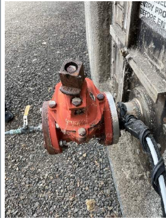
Photo 4-5-1 Broadway - Ultrasonic Level Sensor
