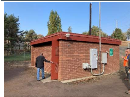
Photo 4-3-25 North Albany Pump Station
