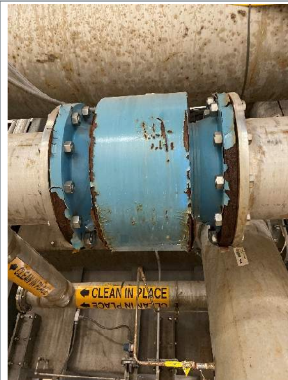
Photo 4-4-24 A&M WTP – Filtrate Flow Meter - Rust
