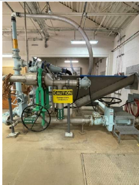
Photo 4-4-23 A&M WTP – RW Intake – Sand Classifier Augers
