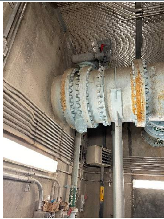
Photo 4-6-2 A&M Intake PS – Low Level Valve
