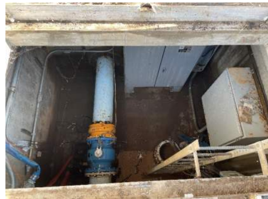
Photo 4-2-12 A&M WTP – Millersburg Meter Vault – Standing Water
