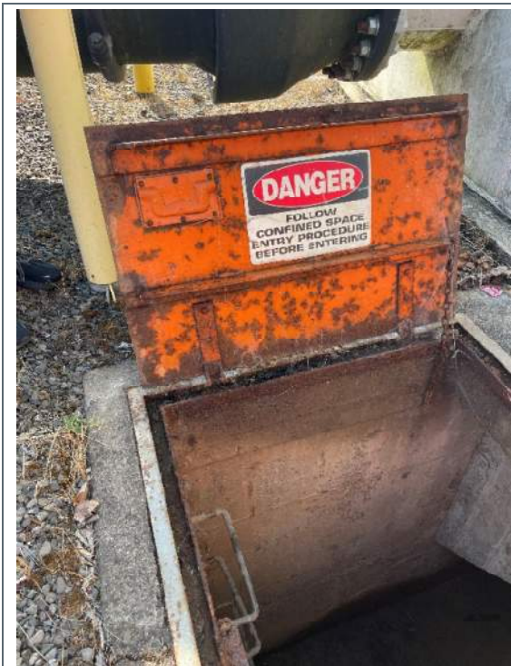
Photo 4-2-5 Maple St – Reservoir Vault - Hatch & Ladder Corrosion
