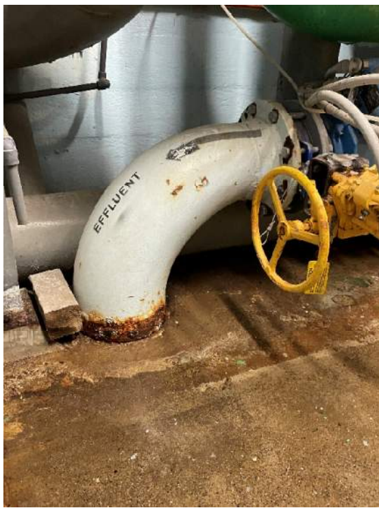
Photo 4-4-16 Vine St – Pipe Gallery – Corrosion & Rust
