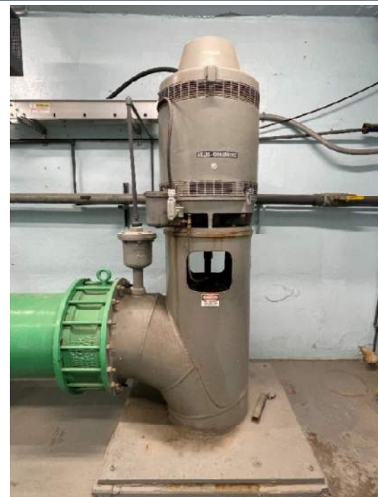
Photo 4-4-14 Vine St – Backwash Pump – Cracked Concrete Base
