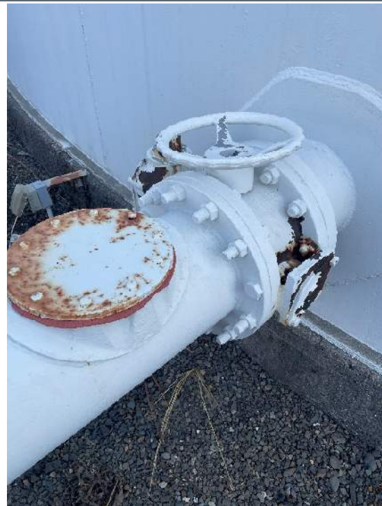
Photo 4-4-11 Queen Ave Reservoir – Rusty Piping
