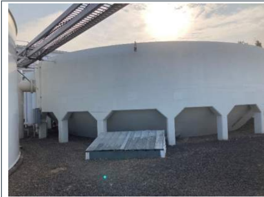
Photo 4-3-13 Vine WTP – Accelerator 1
