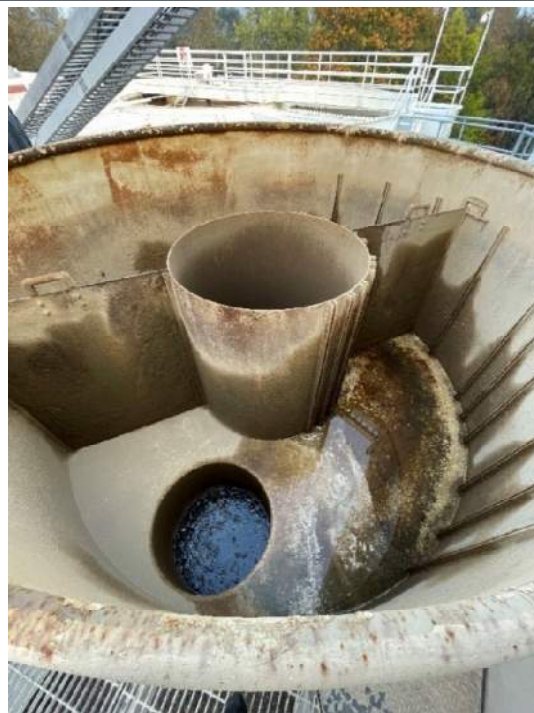
Photo 4-4-15 Vine St – Splitter Box - Rust
