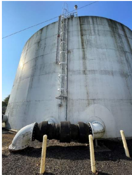
Photo 4-4-6 Maple PS – Reservoir – Worn Coating
