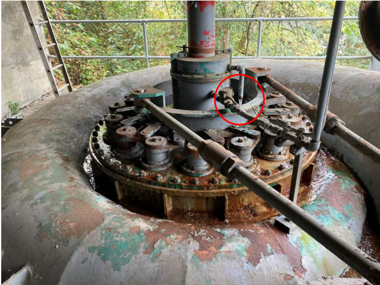
Figure 5. Turbine Bearing Cooling Water Discharge Location. Flooding of Turbine Headcover and Spiral Case is Visible
