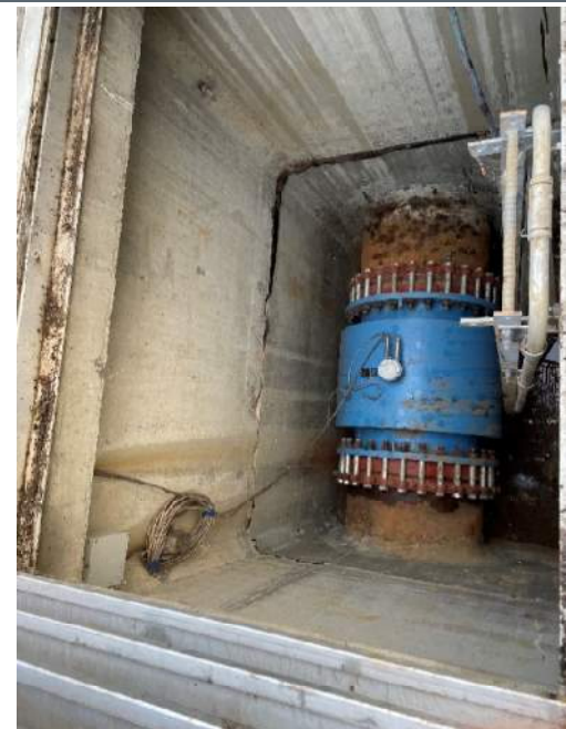
Photo 4-2-4 Broadway – Flow Meter Vault – Standing Water
