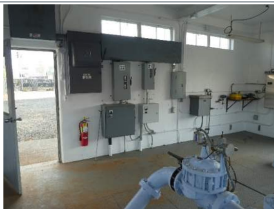
Photo 4-5-6 Queen Ave – MCC NEMA 4
