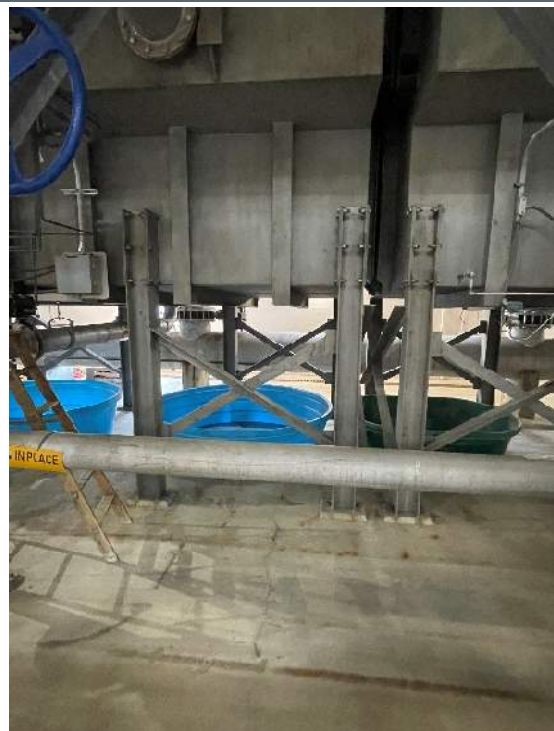
Photo 4-6-3 A&M WTP – Membranes – Plast Blue Pools
