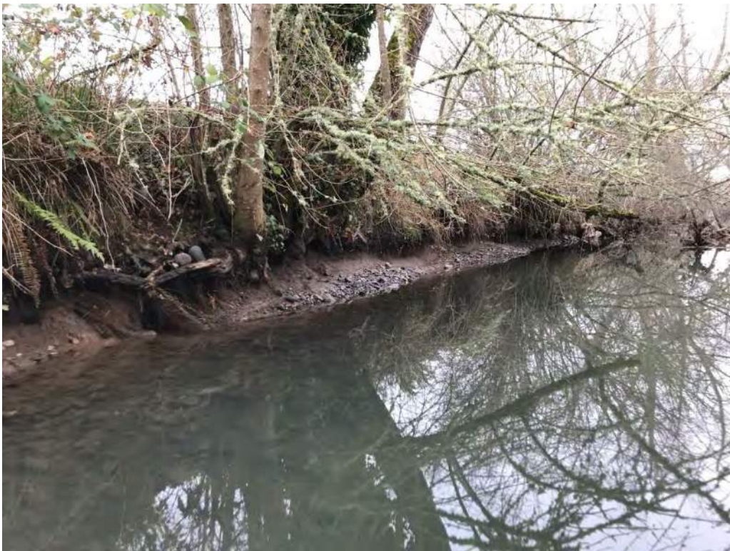
Photo 10. Erosion at the toe of the berm facing northwest.
