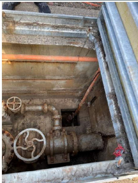
Photo 4-4-9 North Albany – Valve Vault – Rusty Piping
