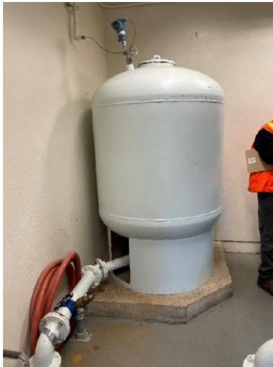
Photo 4-6-7 Valley View PS – Bladder Tank
