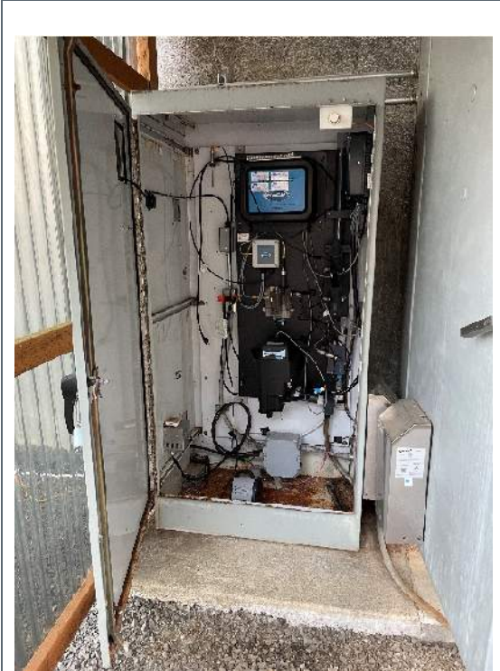
Photo 4-5-3 Broadway - Water Quality Panel
