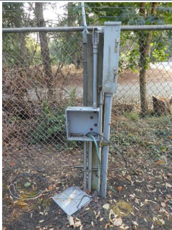
Photo 4-5-8 Valley View – Original 100A Service
