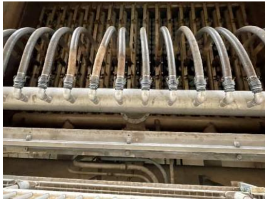
Photo 4-6-5 A&M WTP – Membrane - Hoses
