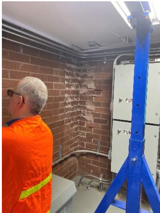
Photo 4-3-31 North Albany Pump Station
