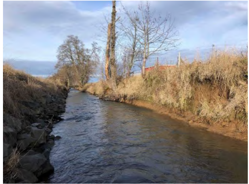
Photo 564: Downstream toward right bank failure
