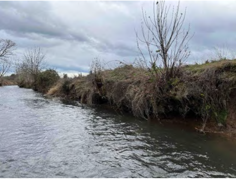
Photo 2968: Left bank upstream of failure
