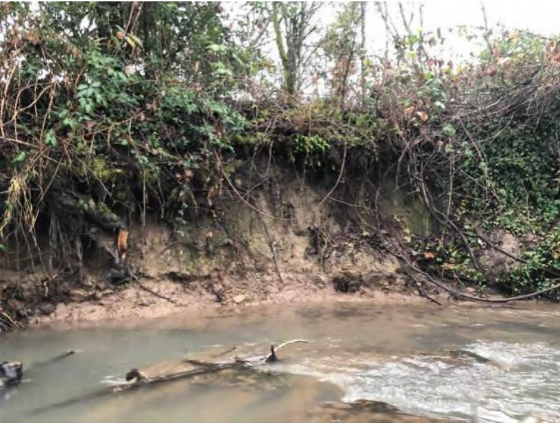
Photo 1044: Left bank failure/erosion
