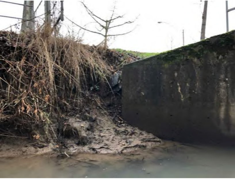
Photo 960: Right bank wingwall erosion
