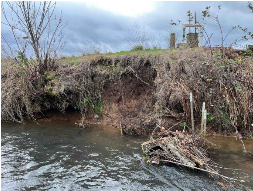
Photo 2966: Original failure (left bank)
