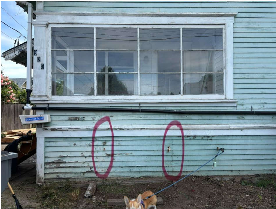
Evidence of step removal
