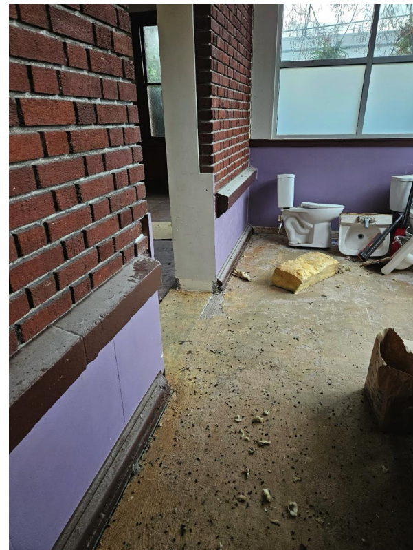
View of interior of annex connection. Existing walls to be restored when connection is removed.
